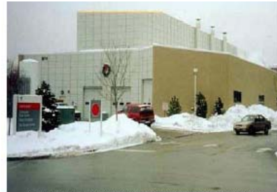
Northwest Community Hospital Central Utility Plant Building. Lower Left: Singe Waukesha Engine.
